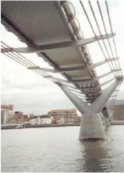
Figure 2. Transverse Arms and Cables
