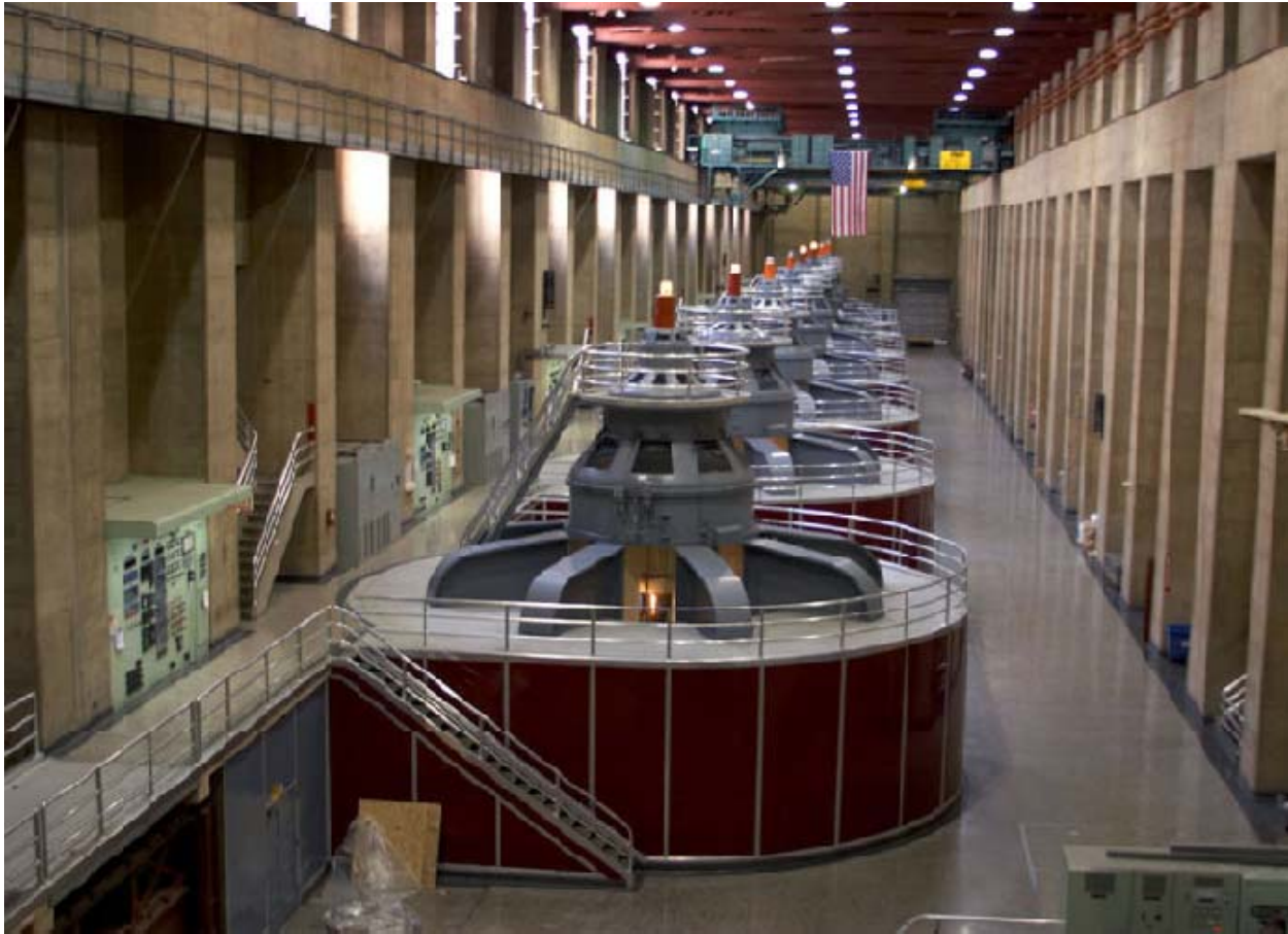
Figure 1. Hoover Dam Turbine Generators (Image courtesy of Wikipedia)
