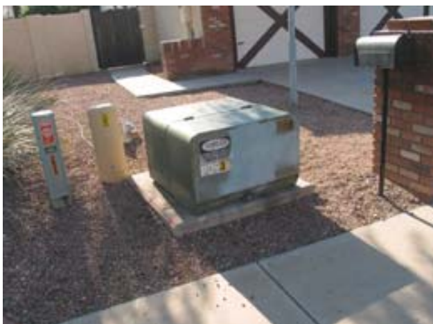
Figure 3. Transformer, Mesa, Arizona
