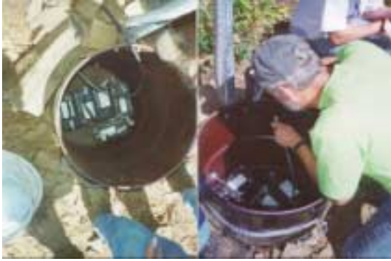
Figure 1. Acoustic Flow Meter Installation
